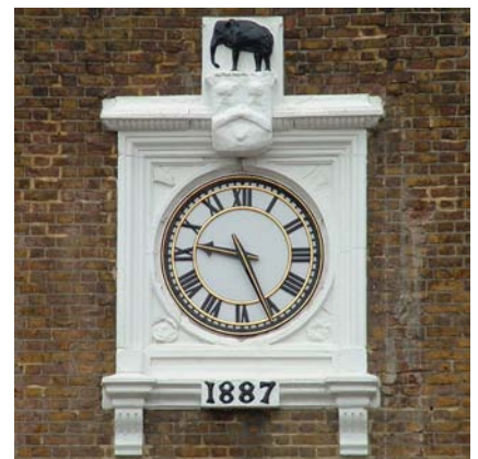
GRP replacement for a corroded cast iron dial, installed in the original surround.
