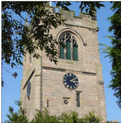
Newly restored church clock dial, cast iron skeleton type with sheet copper backing.
