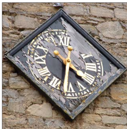
Before: wood dial deteriorated beyond repair.
