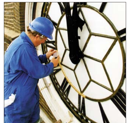
Access to a historic clock tower dial from scaffolding in place for other building work.
