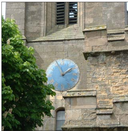
Before: copper church clock dial which has weathered and faded.
