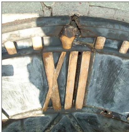
Corroded fixing which has expanded and broken the cast iron dial and stone surround.
